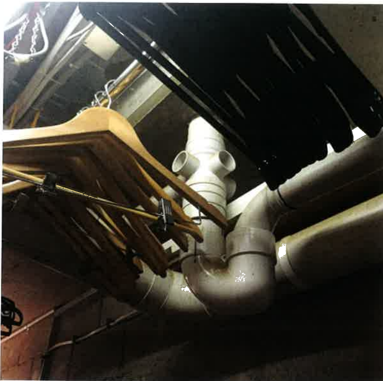
Figure 1 – Intumescent fire collars are required to be post fitted to plumbing penetrations.
