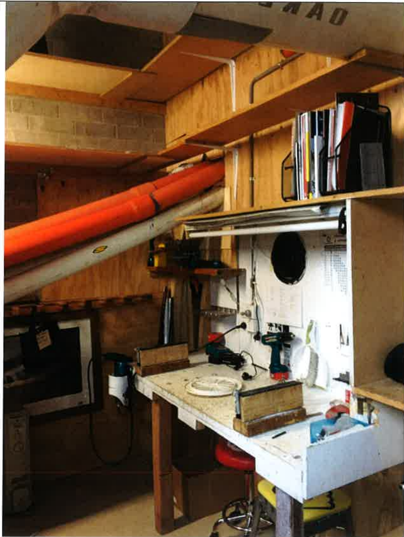
Figure 3 - Electrical conduits located in workshop area.
